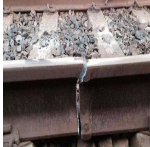
Figure.9 Railway crack on track
